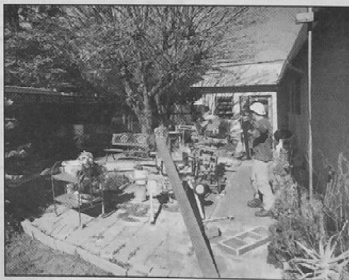
Custom built pieces are fabricated out back while others install them inside the house.
