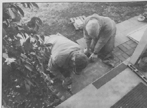
Volunteers work to make front door steps easier to navigate. Photo Credit for all photos: Duncan Cook.
